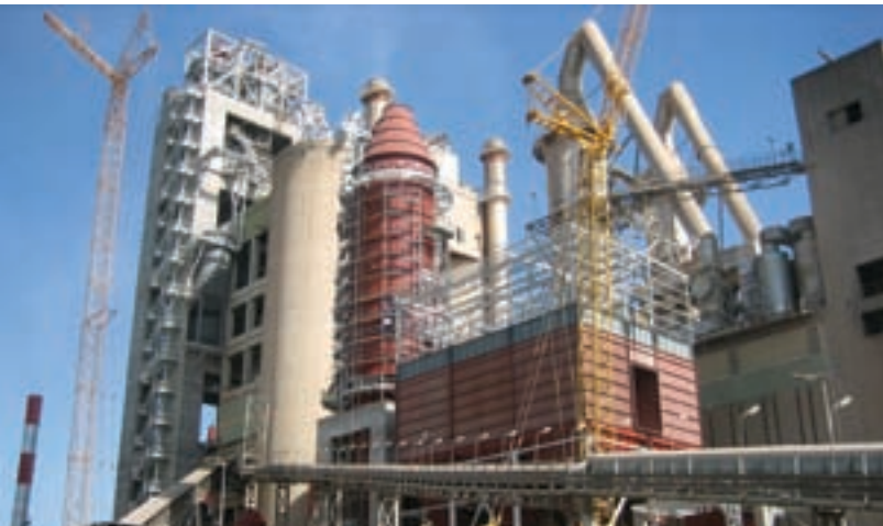
The photos were taken at the Beremend plant between 2007 and 2009
