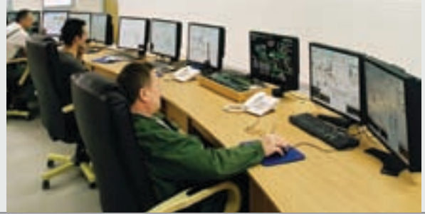
Control panel at the Vác plant
