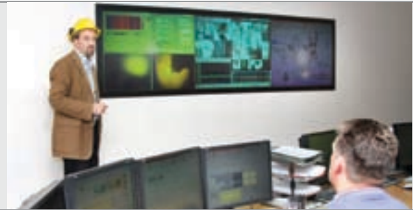
Control panel at the Vác plant
