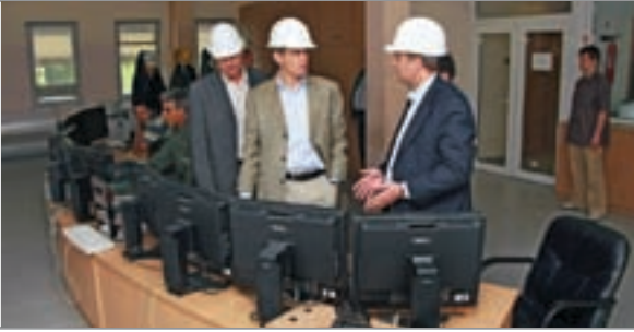
Control panel at the Vác plant
